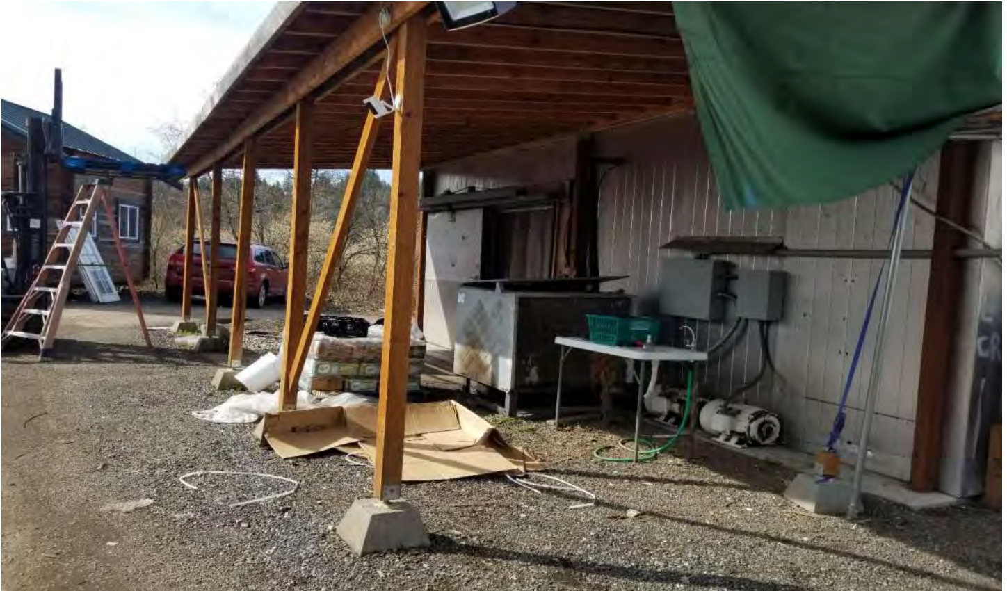
Above: Freezer unit south side of building
