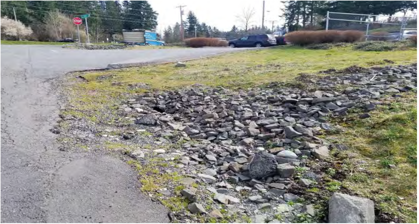
Above: Rip Rap Pad drainage from Renton Maple Valley Road and Parking Lot outfalls here
