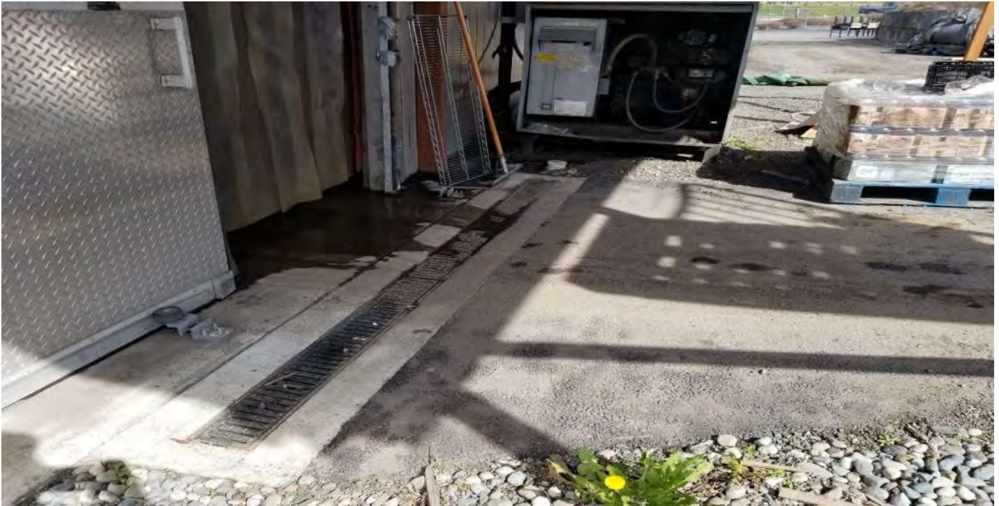
Above: Freezer unit French drain
