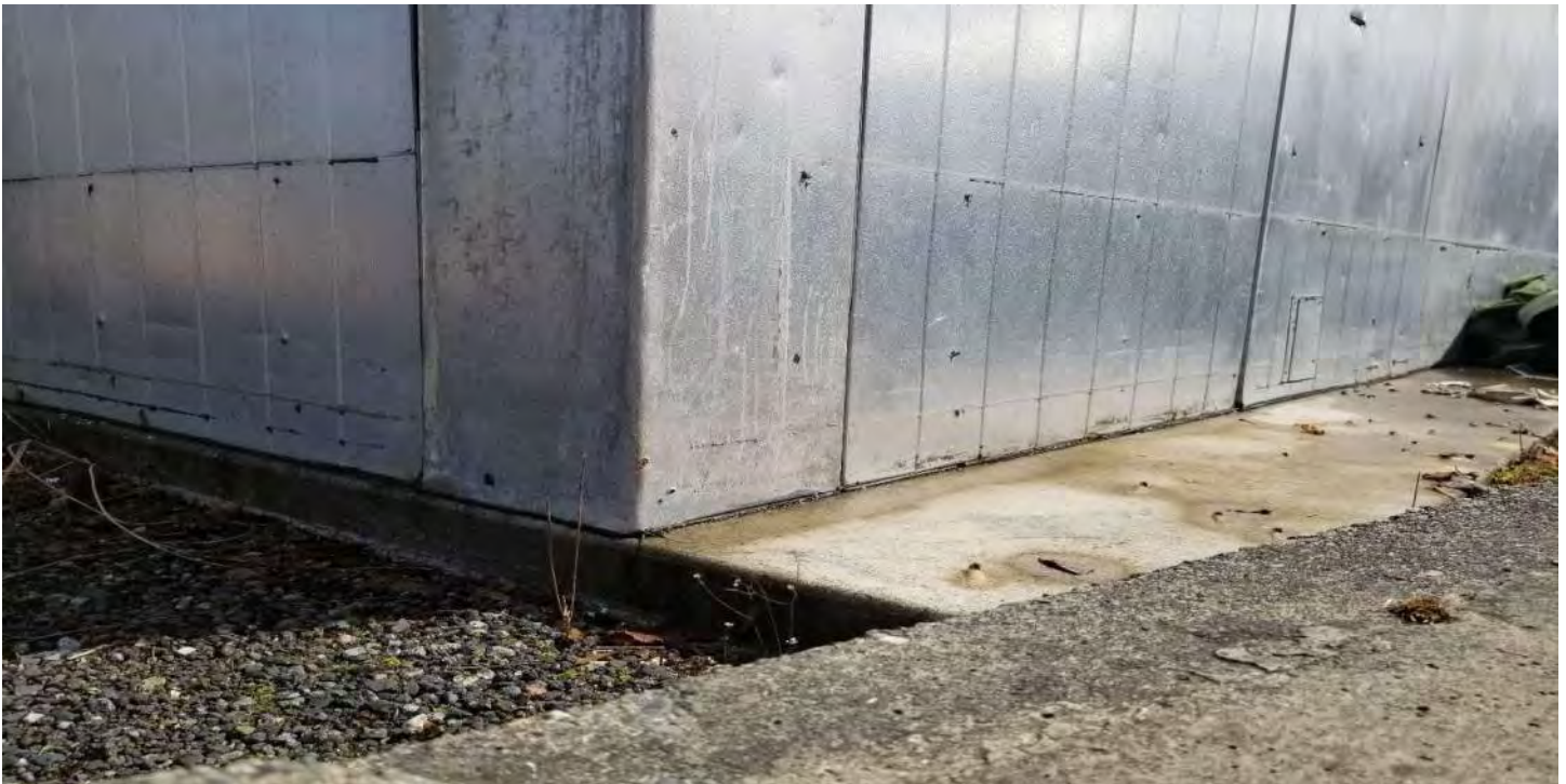
Below: Freezer unit 4" concrete pad below unit
