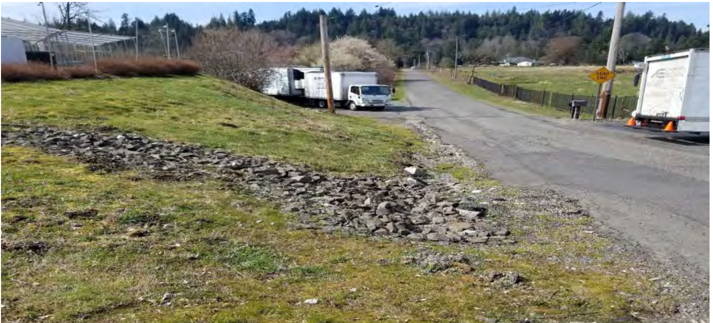
Below: Looking at Rip rap pad where lot drains to as well as CB in eastern parking lot
