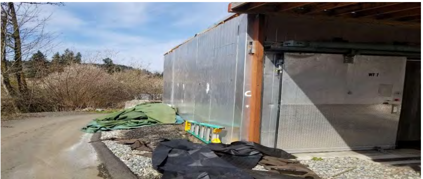
Below: Freezer unit west side of building
