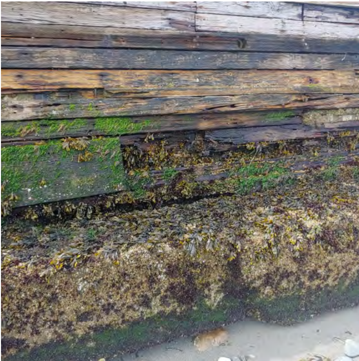
Bulkhead wood degradation and undermining
