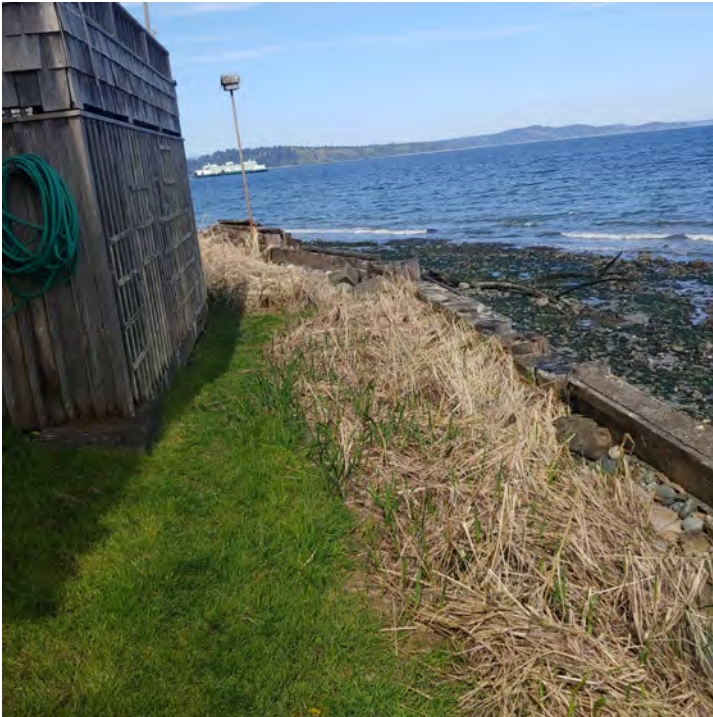
Backfill scour that has been repaired with cobble stone fill and plantings
