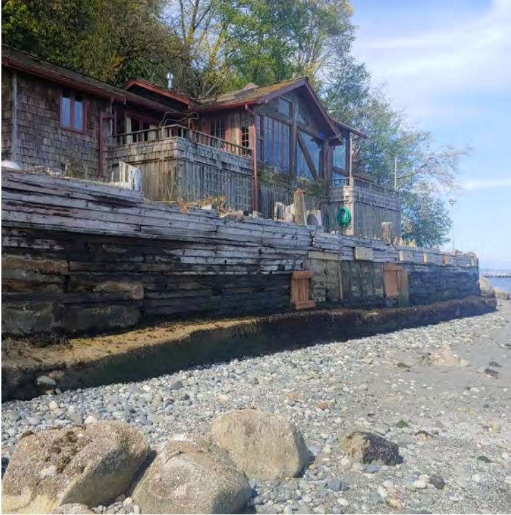
Bulkhead in poor condition with close proximity of primary structure
