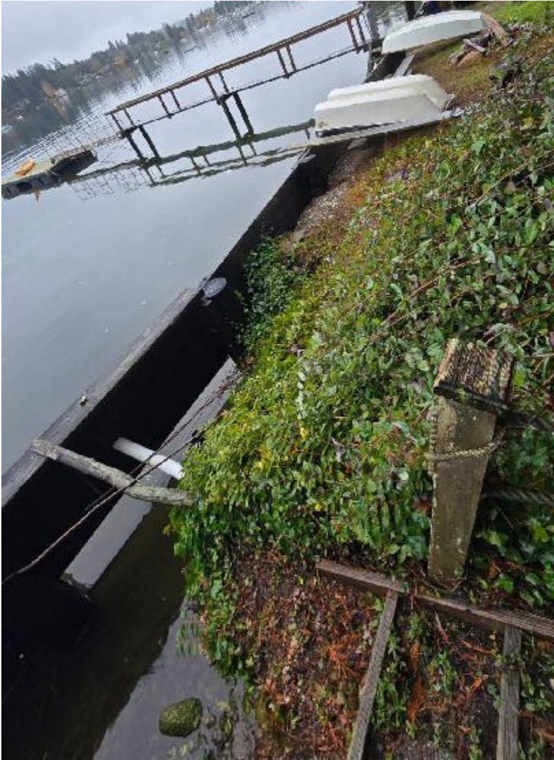
Photo 2: Active Shoreline Erosion Behind Bulkhead to South Beyond Bulkhead Failure
