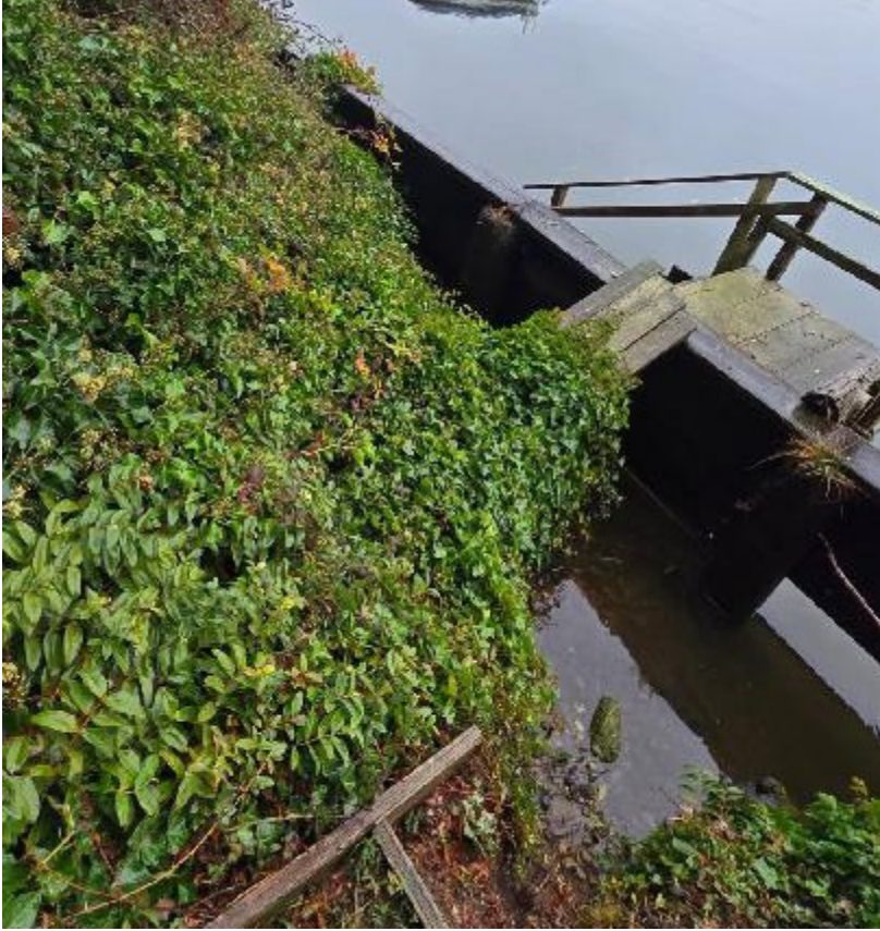
Photo 3: Shoreline Erosion Behind Bulkhead to North Beyond Bulkhead Failure
