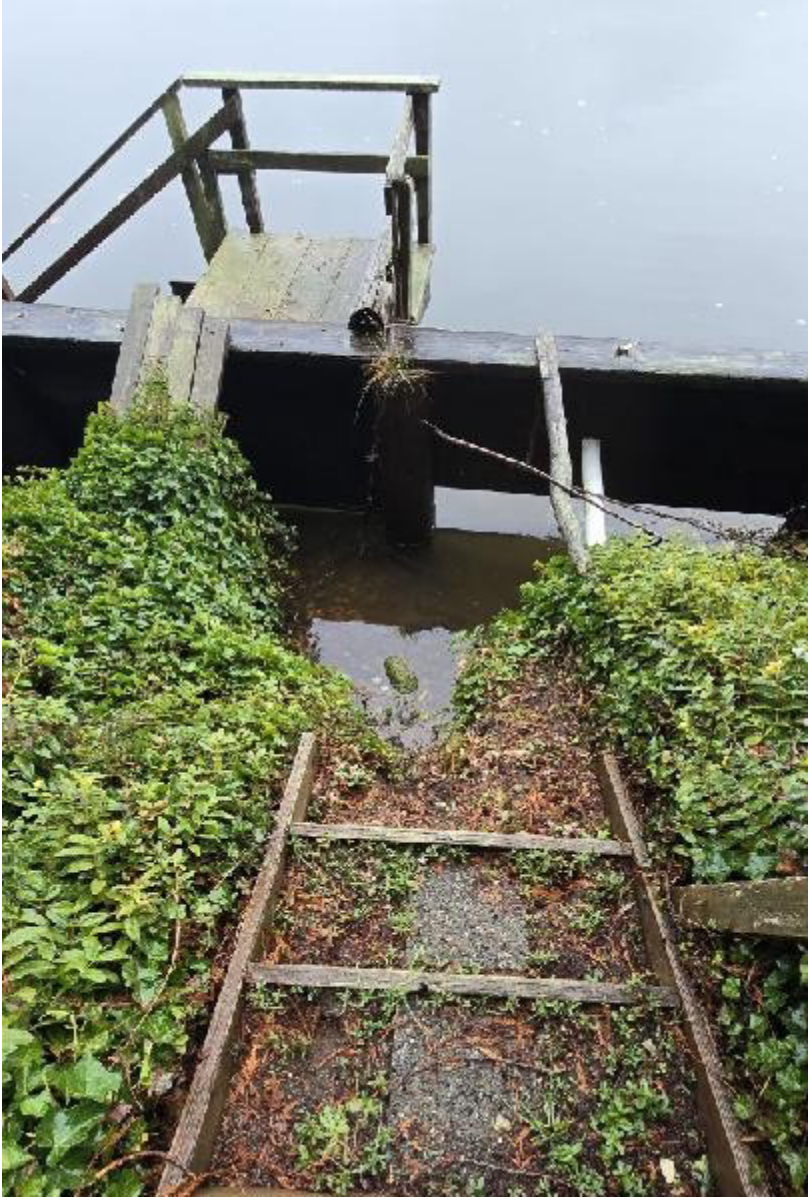
Photo 1: Failed Timber Bulkhead w/ Backfill Erosion
