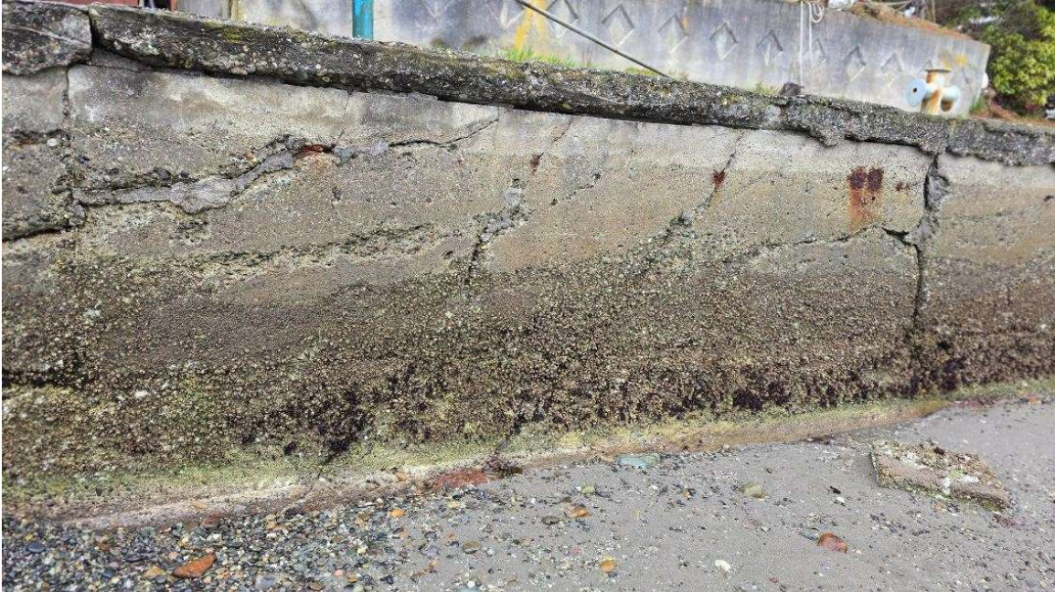
Photo 1: Bulkhead Cracking and Reinforcement Bleeding.
