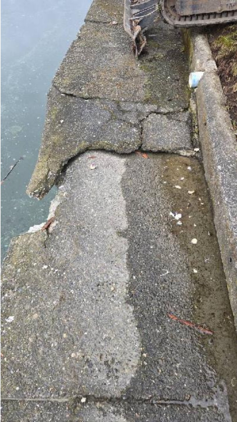
Photo 4: Failing Bulkhead Cap & Slight Backfill Erosion
