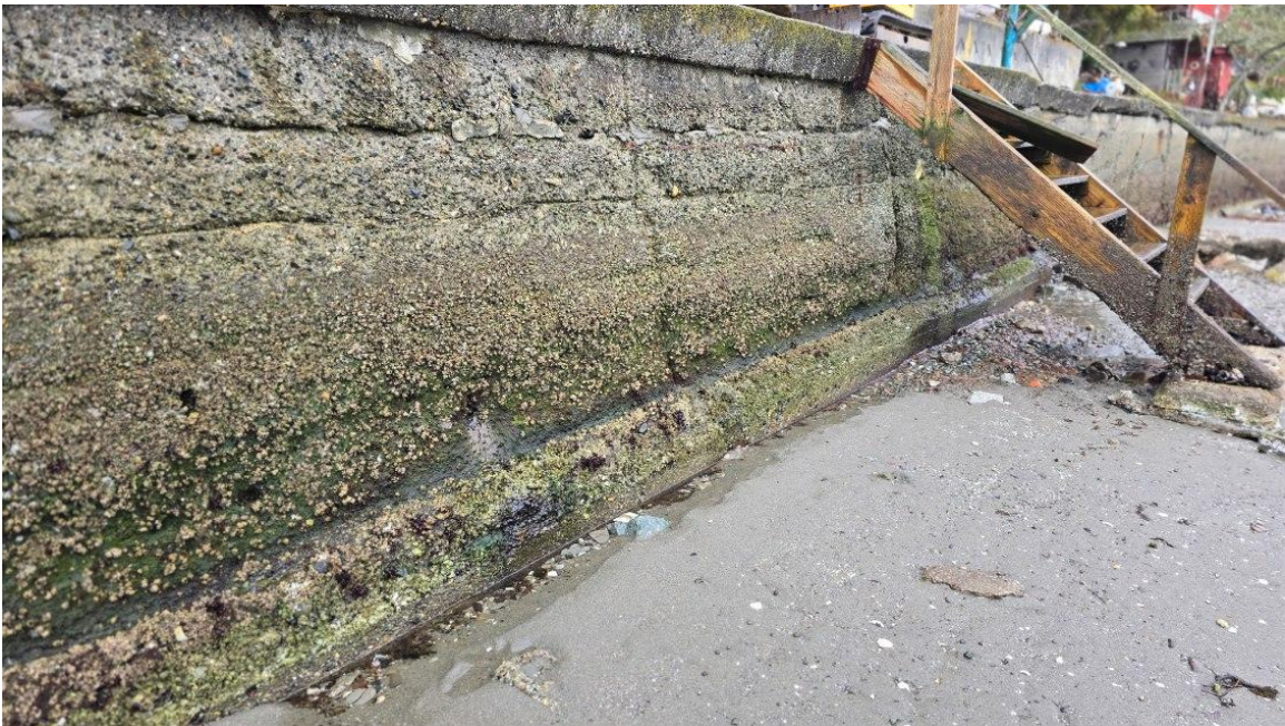
Photo 2: Bulkhead Concrete Degradation.
