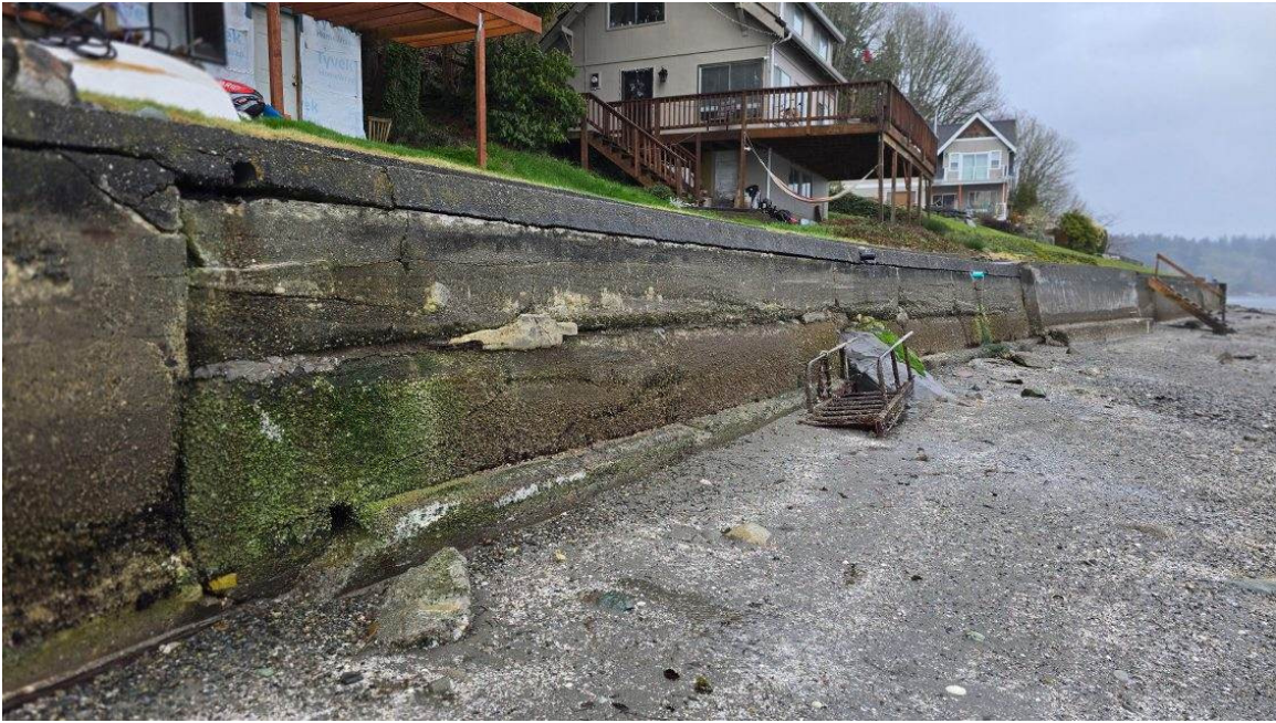
Photo 3: Bulkhead & Beach Erosion
