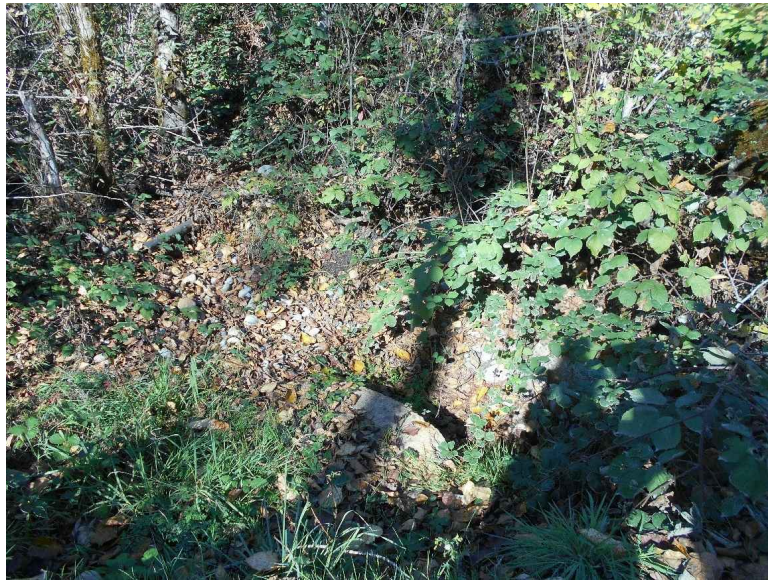
PHOTO 1: CONCRETE CHECK DAMS CONSTRUCTED AS PART OF THE ENGINEERED CHANNEL. LOOKING NORTH, NORTH OF THE SOUTHERN ACCESS ROAD, CONCRETE CHECK DAMS DIRECT-FLOW INTO THE CULVERT LEADING TO THE MAIN INFILTRATION AREA.
