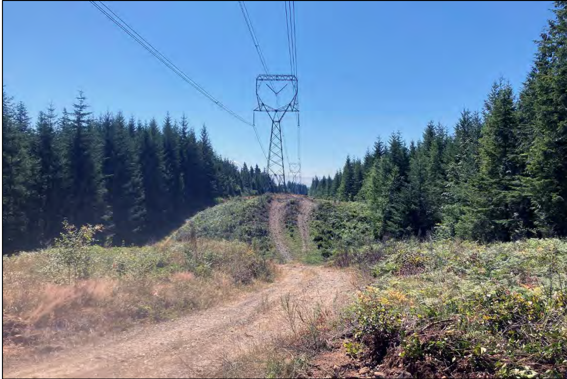
Figure 17. Overview in area M-3 along the Raver-Paul No. 1 Transmission Line; view south.
