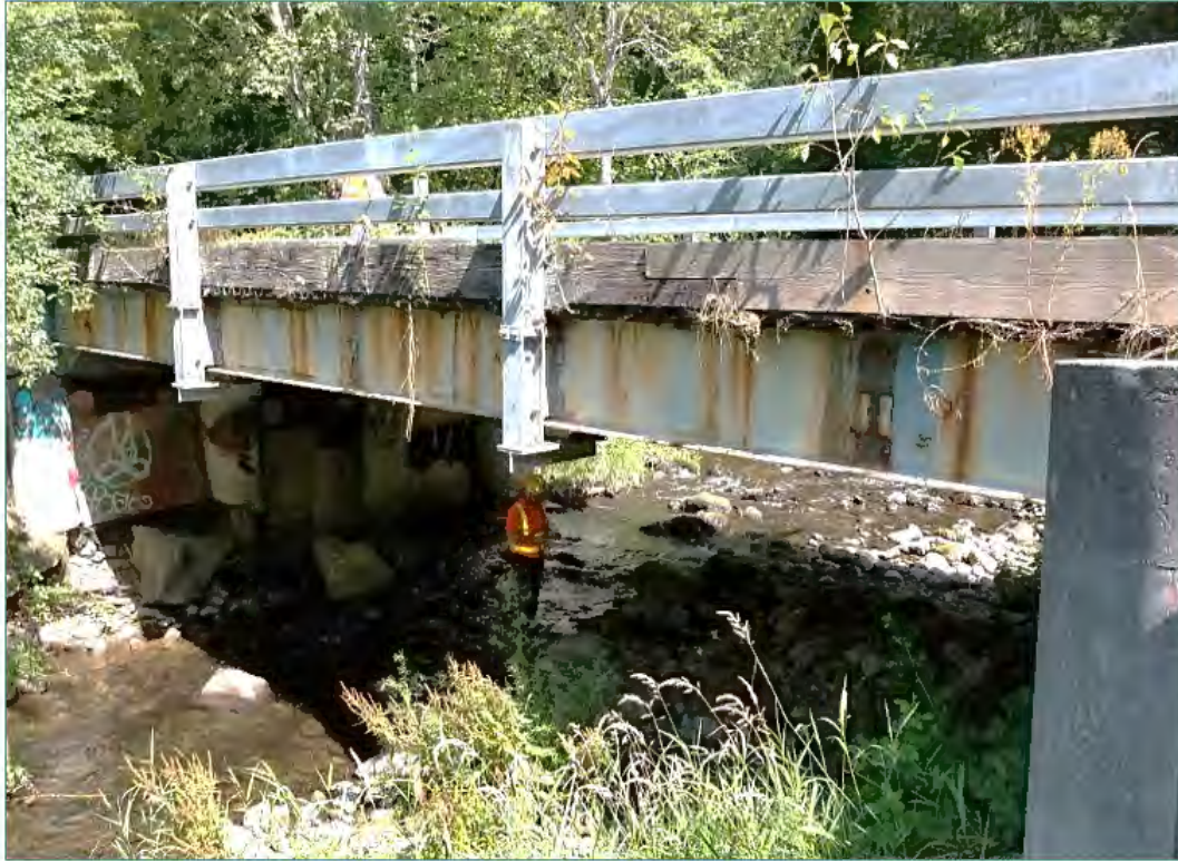
Figure 17: Boise X Connection Bridge No. 3055A - Deteriorating steel girders and timber piles
