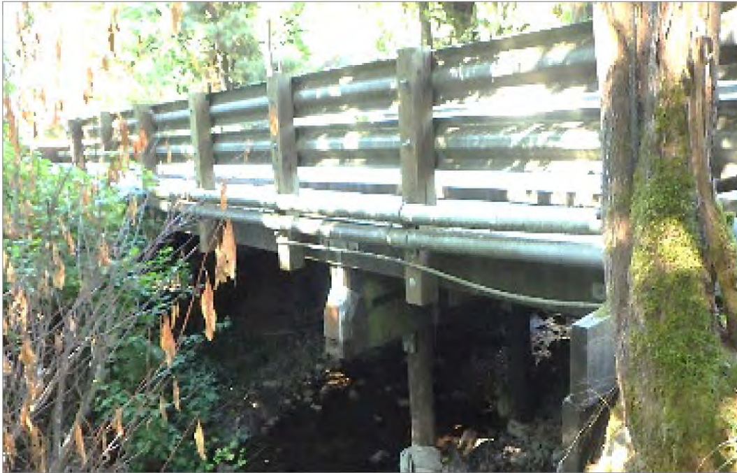
Figure 18: Fifteen Mile Creek Bridge No. 493C - Deteriorating timber superstructure and substructure.
