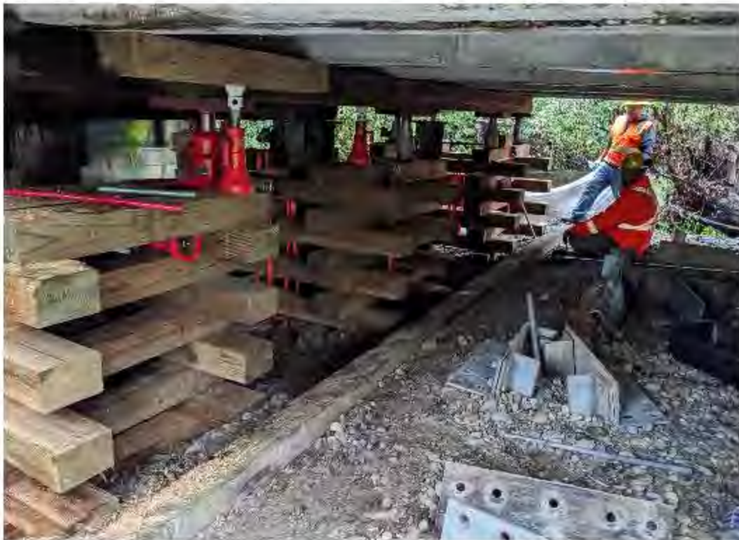
Figure 7: Issaquah Creek No. 83B - Hydraulic jacking up bridge to replace timber cap.
