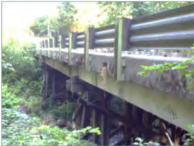
Figure 13: Upper Tokul Creek Bridge No. 271B – Deteriorated structure before replacement
