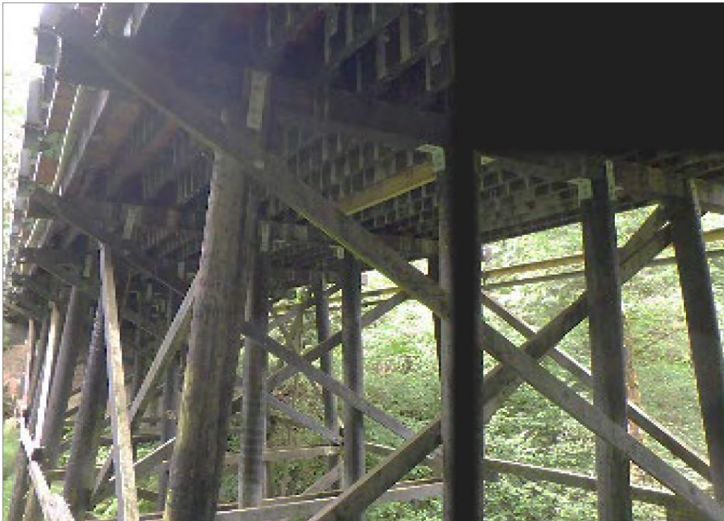
Figure 16: Ames Lake Trestle No. 1320A – Deteriorating timber stringers, caps, and piles.
