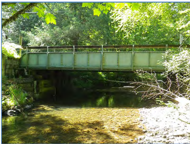
Figure 11: Coal Creek Bridge No. 3035A – Deteriorated structure before replacement
