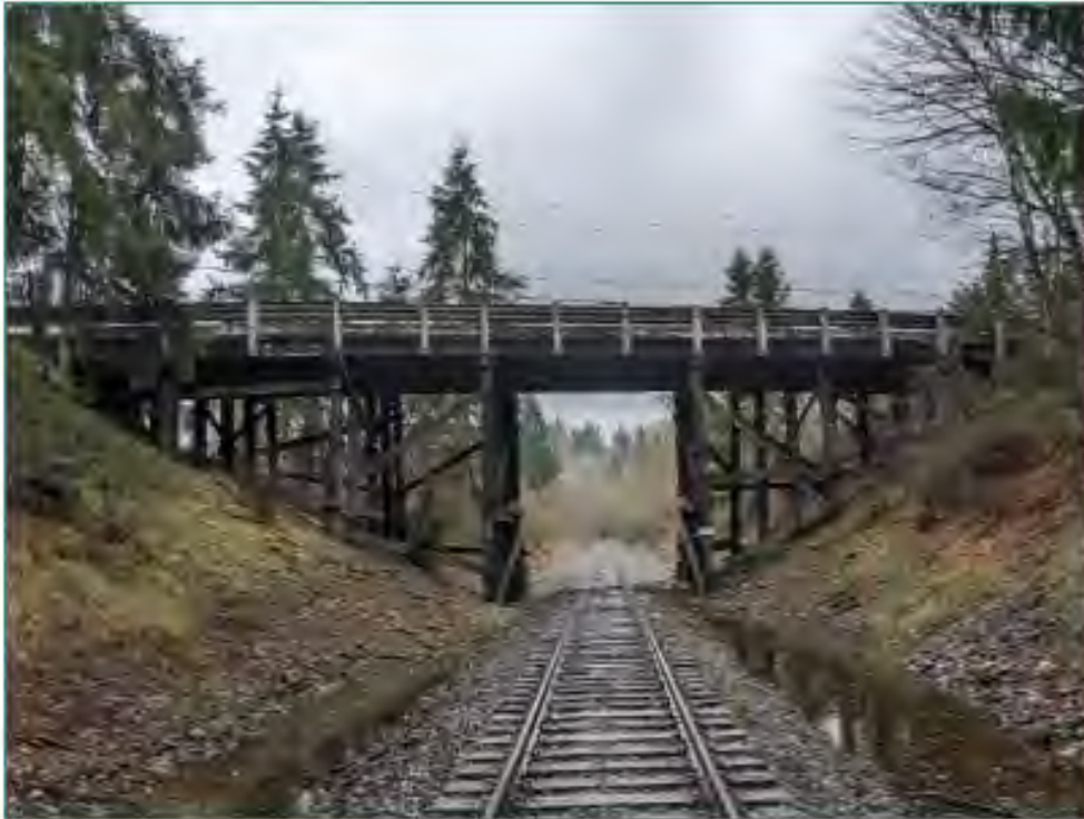
Figure 20: Berrydale Overcrossing Bridge No. 3086OX – Looking south over the BNSF rail line.
