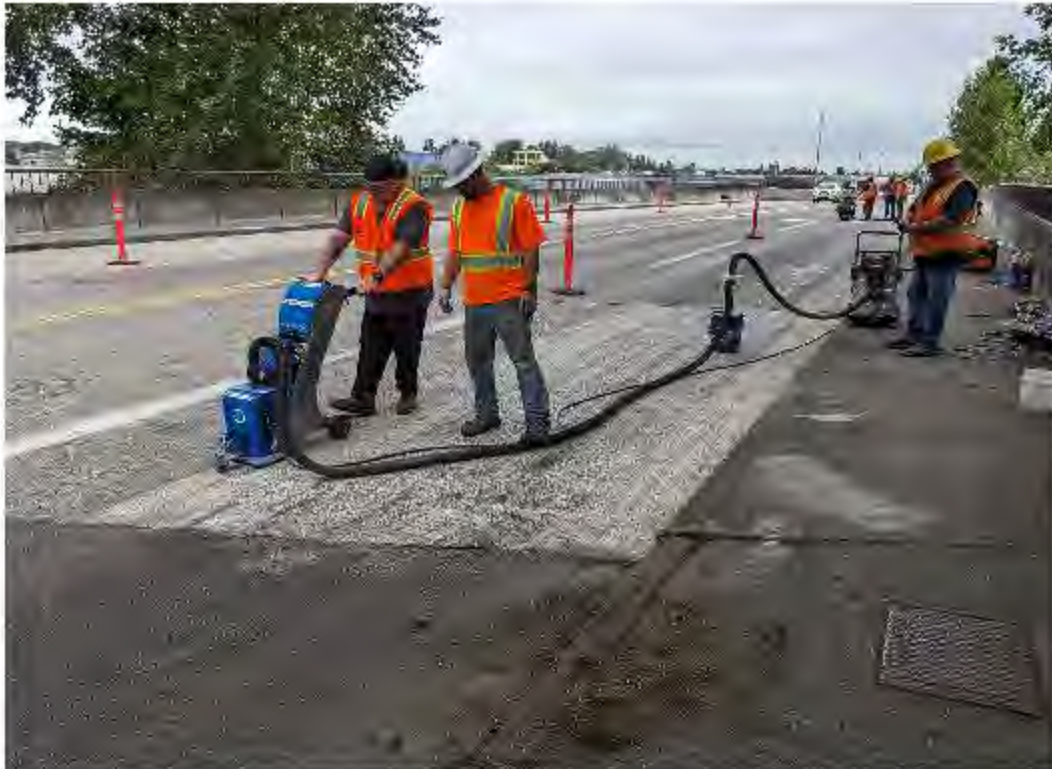
Figure 8: Green River Bridge No. 3216 - Shotblasting bridge deck prior to deck sealant application.
