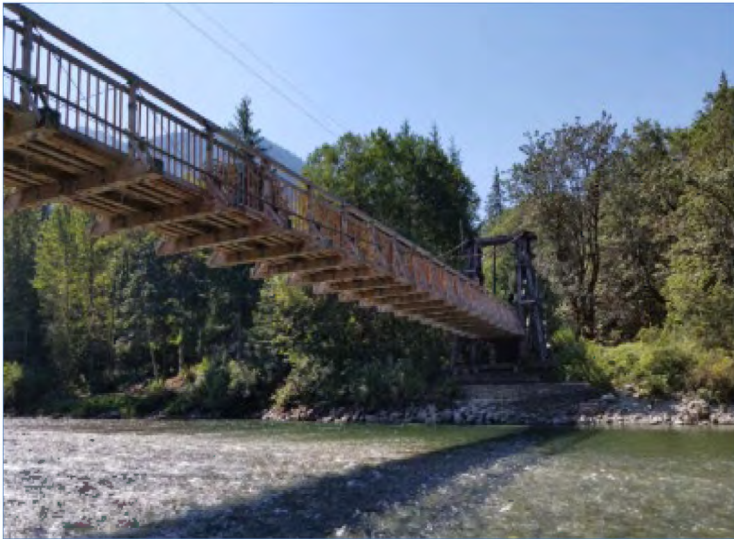
Figure 15: Baring Bridge No. 509A – South tower and timber truss of suspension bridge spanning the Skykomish River
