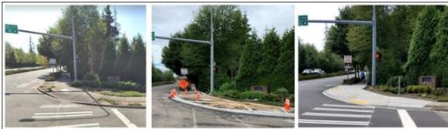
Photos show the Before, During, and After of a finished curb ramp improvement project at NE Novelty Hill Road and 238th Place NE.
