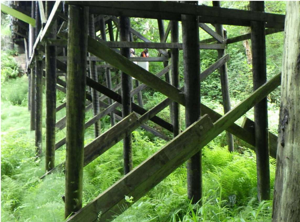
Decaying creosote-treated timber piles
