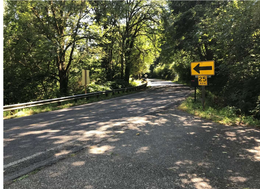
Poor visibility for oncoming traffic
