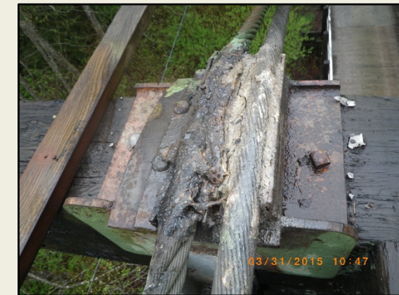
Rusted cables at the top of towers.
