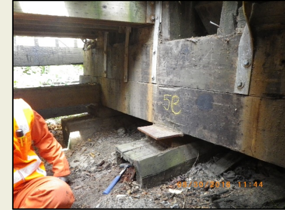
Crushed timber sill support under Cap 5.
