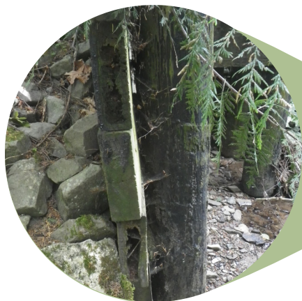
Decaying timber support structure
