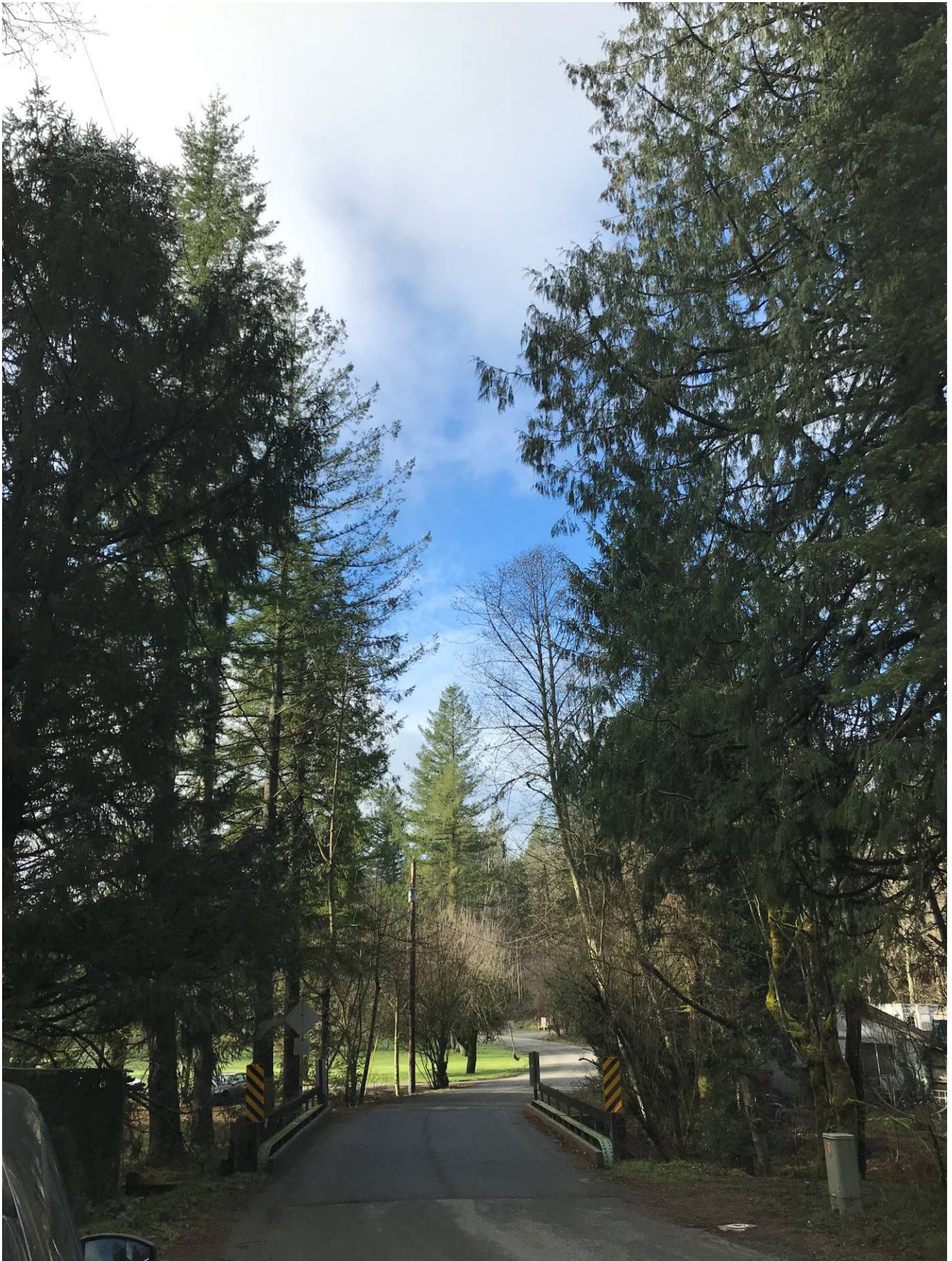
Looking west on SE Lake Walker Road at the bridge deck and surrounding tree canopy vegetation
