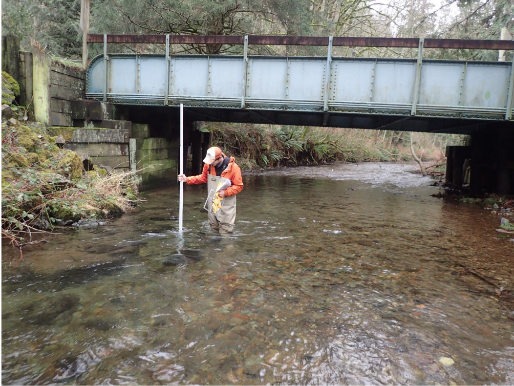
Looking downstream, thalweg between LB culvert and bridge. Rip Rap on LB. Max depth about 2 feet. (Photo K)
