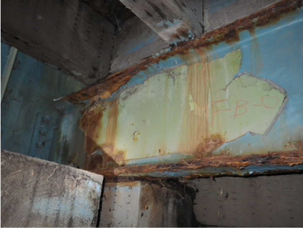
Figure 3-8: Deterioration of Steel Floor Beams
