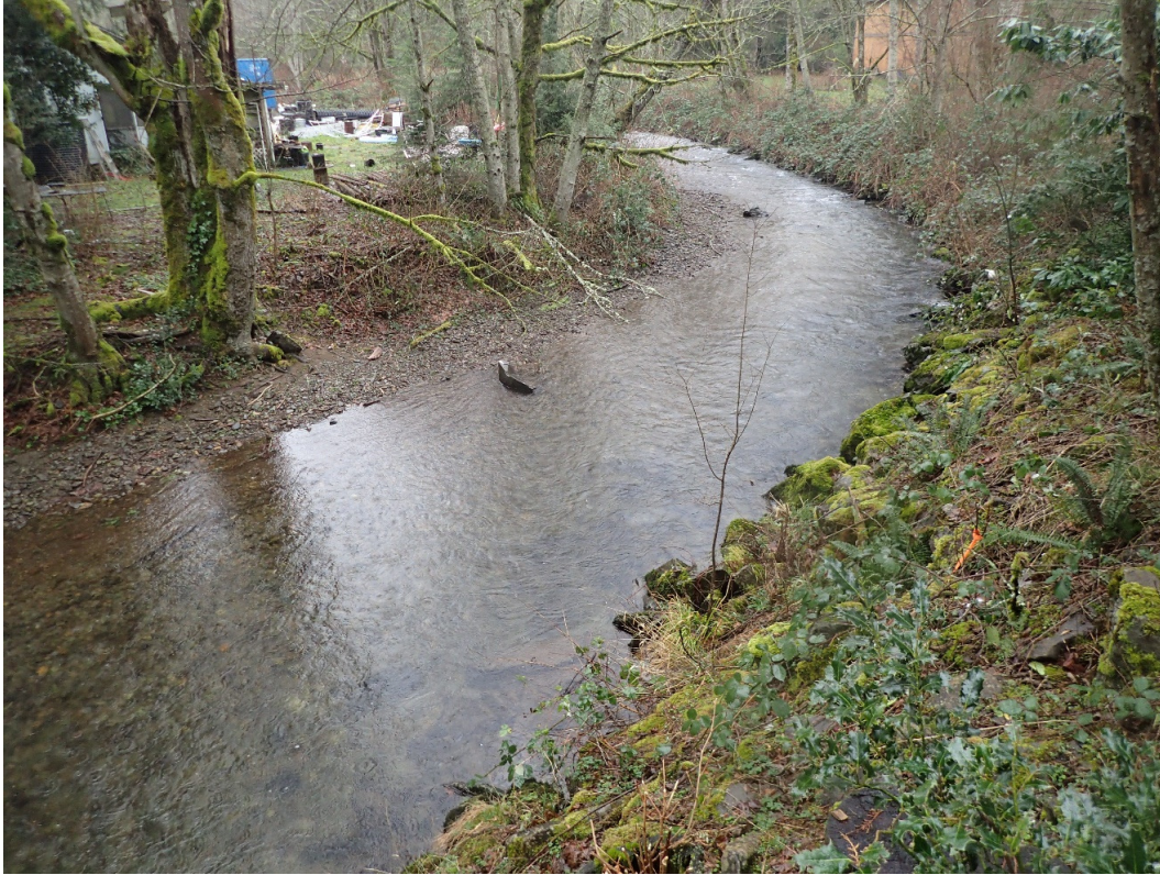
Looking upstream from LB end of bridge at rip rap bend (Photo O)
