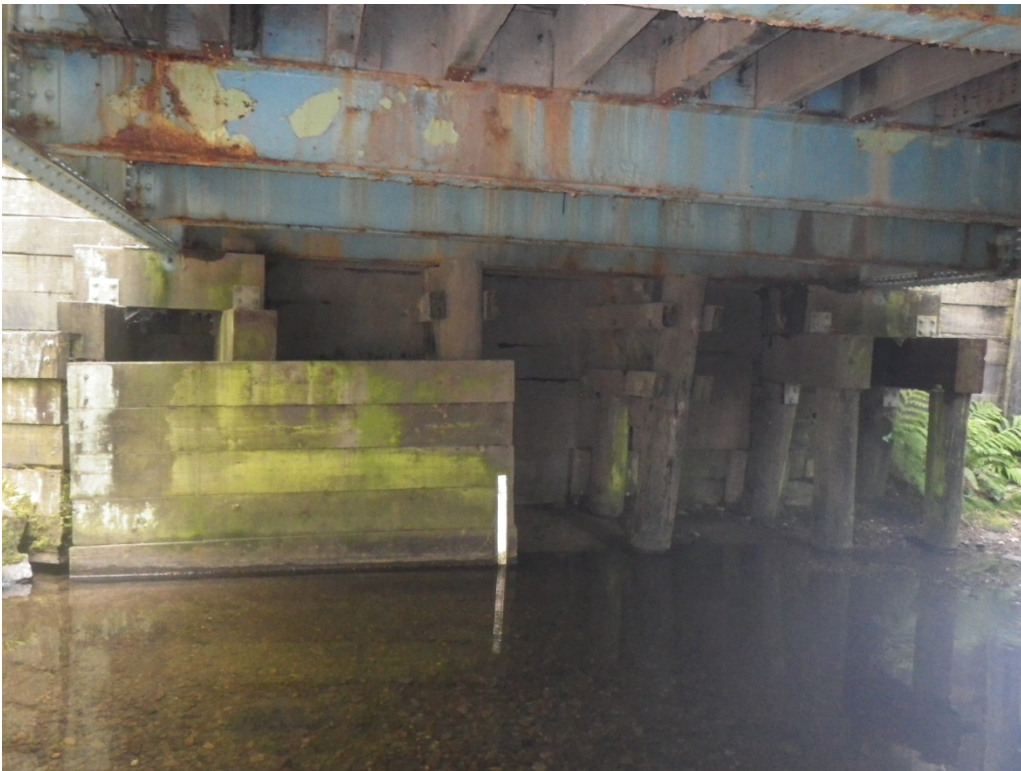
Figure 3-9: Timber Piling & Bulkheads with Repairs
