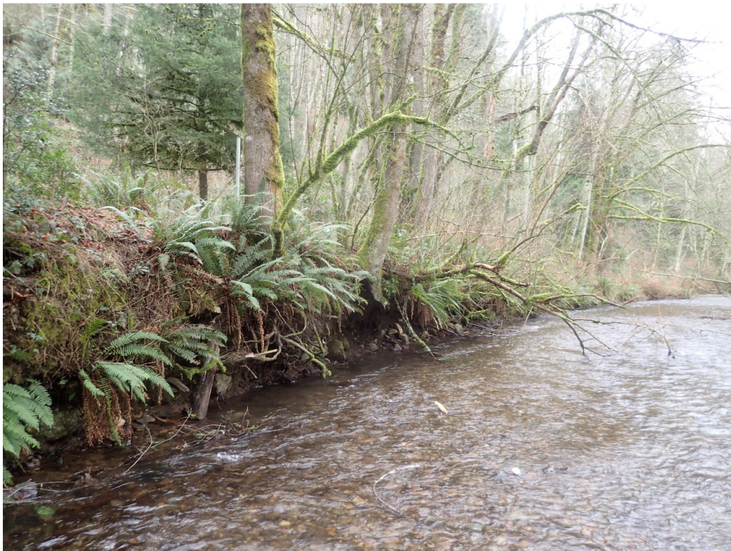
Looking downstream at undercut LB just downstream of bridge (Photo H)
