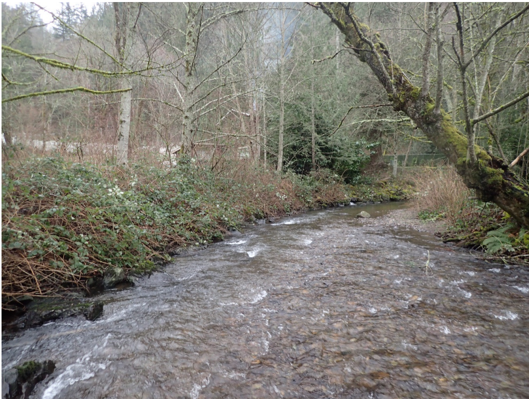
Looking downstream at bend upstream of bridge. The riprap is on the LB in distance, and on the RB at the section where photo is taken. (Photo L)
