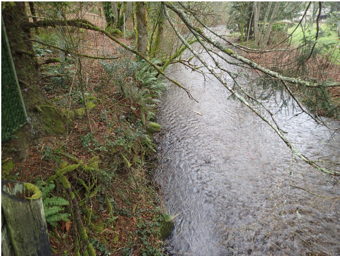
Looking downstream from LB end of bridge at undercut LB. (Photo P)
