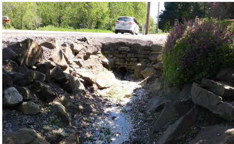
Crews will be replacing the small culvert shown here directly below the white car on 284th Avenue SE.
