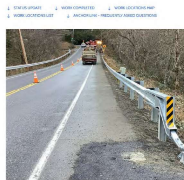
Photo: K. 2023 - Guardrail installation project - Route 20 (SR 20) East from SR 160 to SR 161 at SR 16
