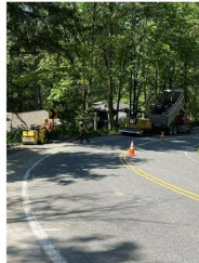
Photo: K. 2023 - Guardrail installation project - Route 20 (SR 20) East from SR 160 to SR 161 at SR 16
