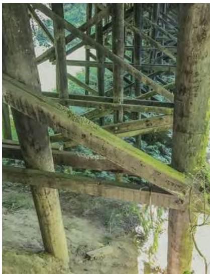
Creosote-treated timber piles are decaying.
