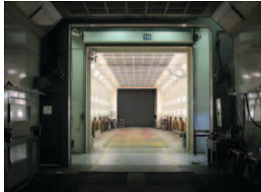
Lighting efficiency retrofit in a painting booth at a Metro Transit bus base
