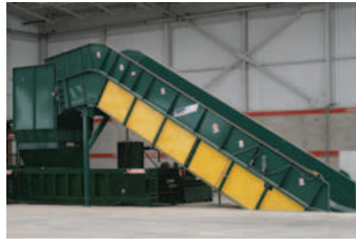
Paper recycling infrastructure at the Bow Lake Recycling and Transfer Station
