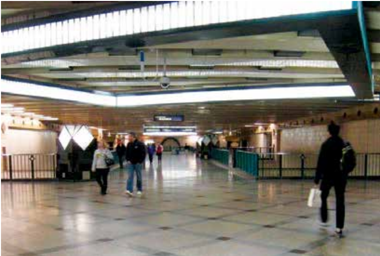
Energy efficient lighting upgrades in the DSTT – Westlake Station
