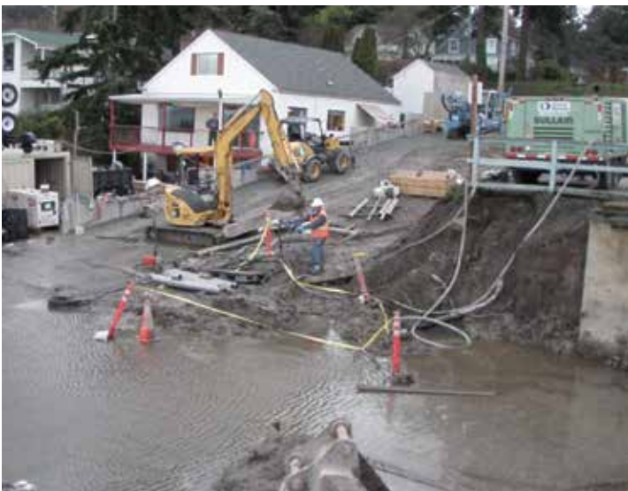
This photo shows just minor damage of the construction site as a result of a record high tide. Damage would have been much worse if the construction crew hadn't accounted for sea-level rise. Work started again within hours and there was no loss of equipment.
