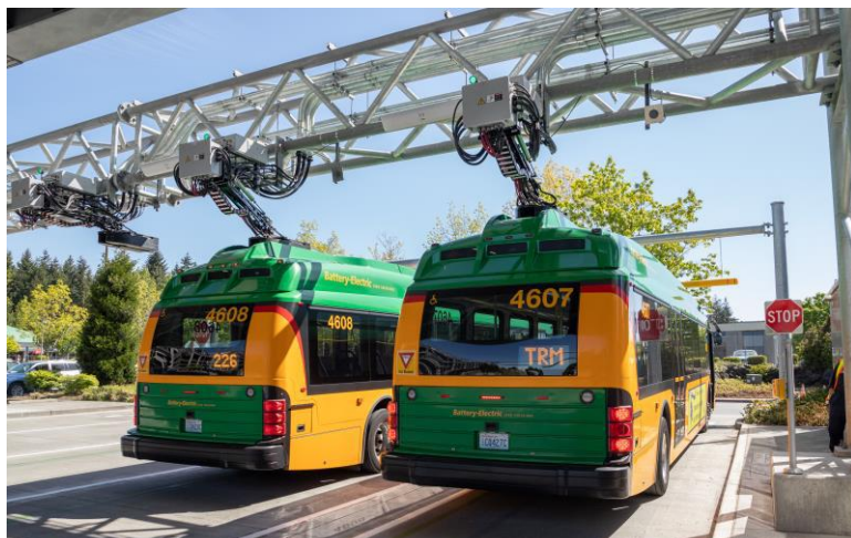
Figure 3. Current Gantry Charging Structure at Eastgate Park-and-Ride
