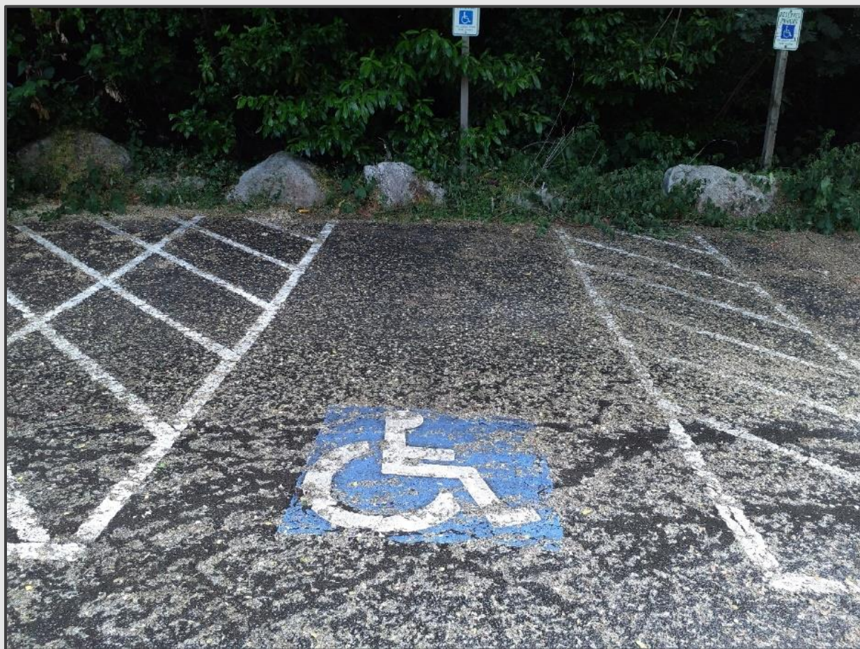
Figure 8: Excessive slopes in parking area
