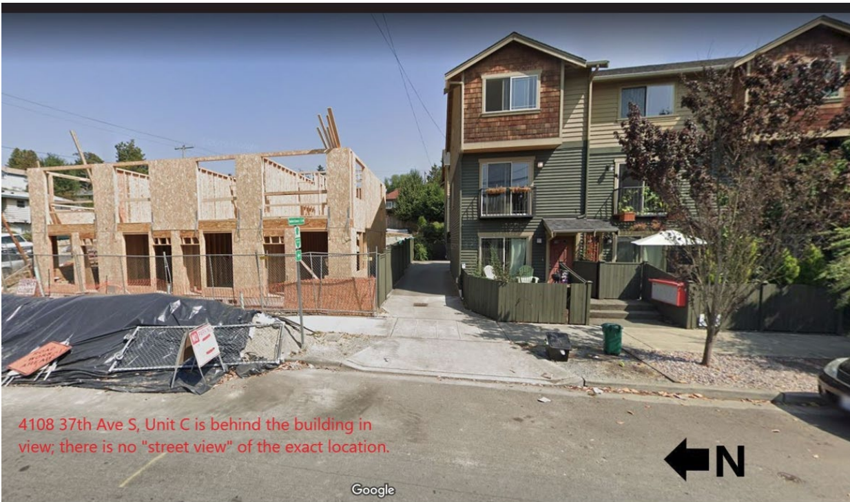
Figure 5 - Photograph of 4104 37th Ave S (under construction) and the driveway between the two buildings.
