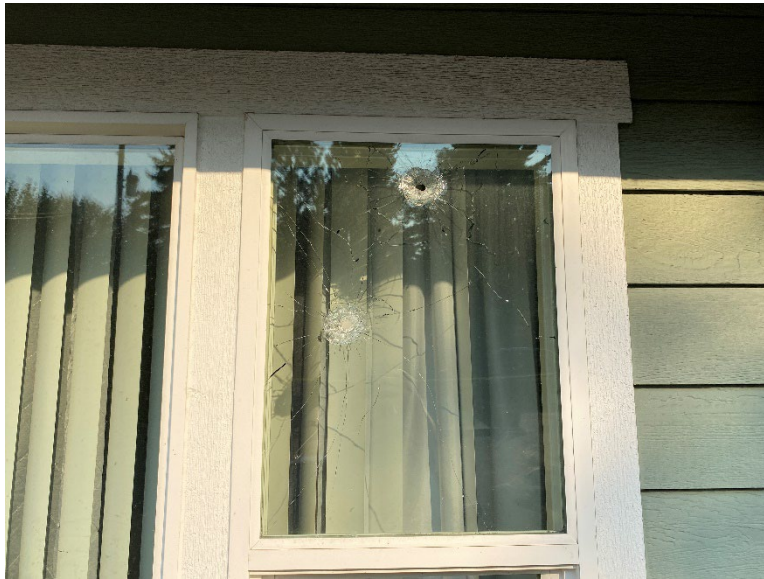
Figure 2 - Bullet defects in Unit A's window.
