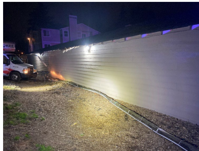
Figure: Photos of damage subject Reilly caused to the retaining wall and building roof.
