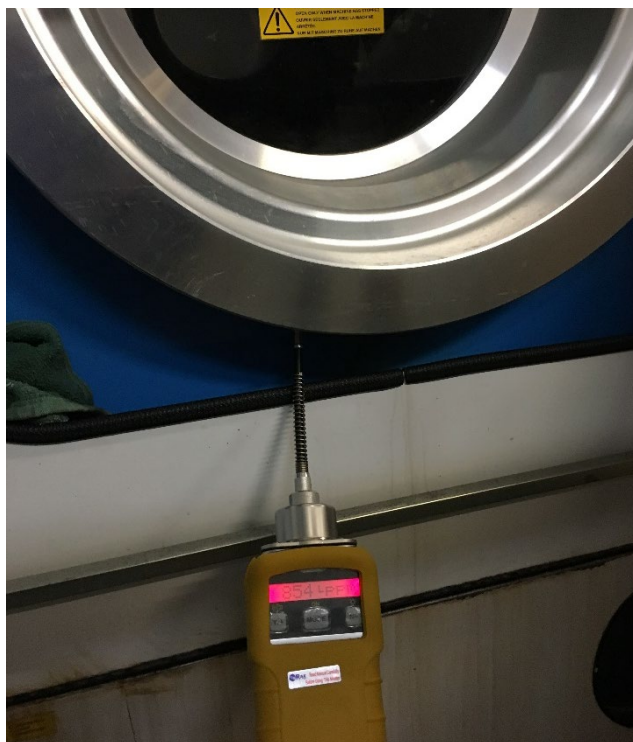
Figure 8. PERC leakage at a loading door Note the visible stains below the door, indicating PERC leakage, and the rag (to the left) used to catch drips. The PID reading is 854 ppm.
