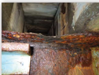
We are losing sections of steel.
