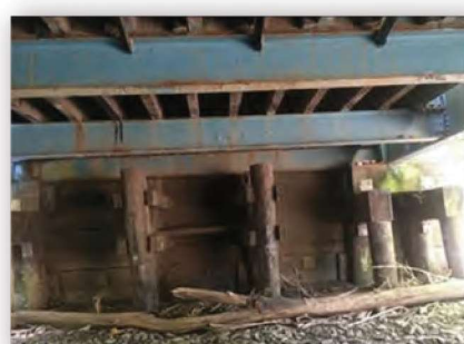
The 63-year-old creosote timbers are rotting.
