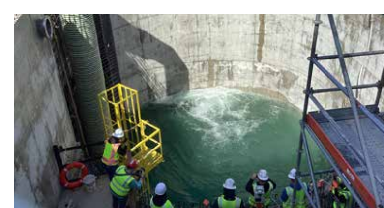
The Ship Canal Water Quality Project is a joint effort between King County and Seattle Public Utilities. The project will capture and store 29 million gallons of polluted water during heavy rains. An underground storage tunnel is being built to hold the stormwater and sewage until there is room to send it to the West Point Treatment Plant. It will control four CSO outfalls for the City of Seattle and two King County outfalls at 3rd Ave W and 11th Ave NW. Construction is continuing.
