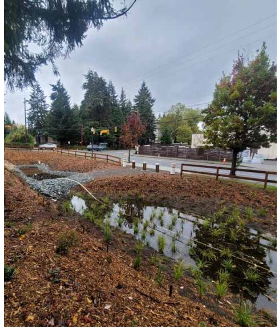
AFTER: Looking north from the center of the project site - sedimentation pond and northern bioretention cell filling with stormwater runoff.
