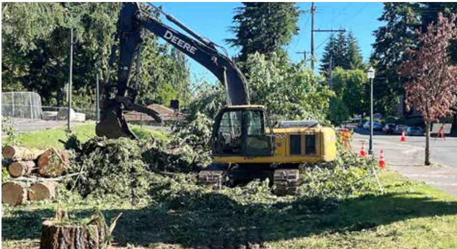
CONSTRUCTION: Looking north from the center of the project site - clearing and grading.
