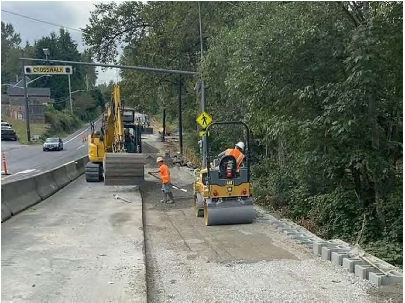
Sept. 23, 2022 – The new sidewall and shoulder is compacted before the new sidewalk is installed.
