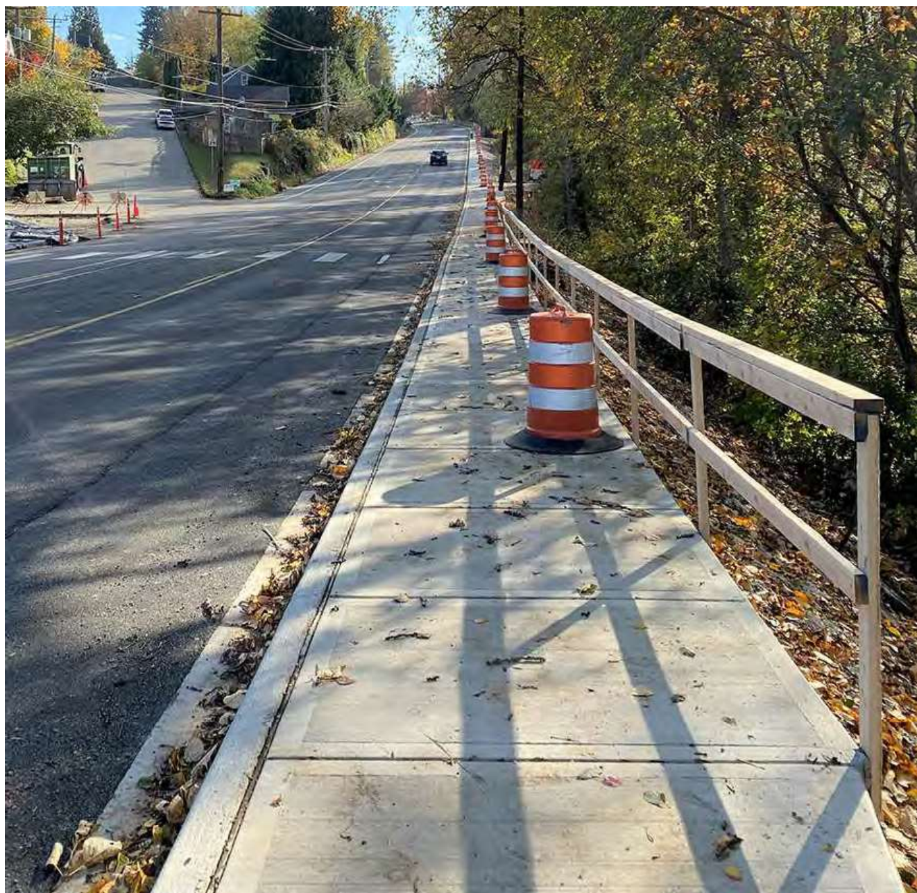
Nov. 10, 2022 – The finished bike lane, sidewalk, and gutter stretch down the west side of Renton Avenue S.
