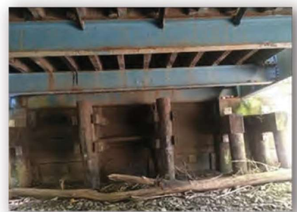
The 63-year-old creosote timbers are rotting.
