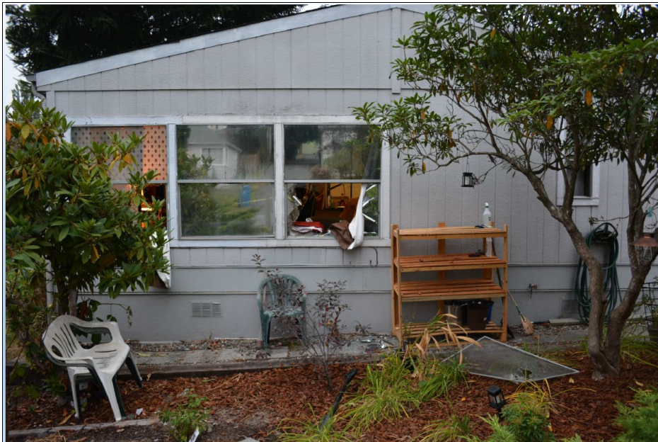
Figure 9- Side 2 of home, showing Peppan’s bedroom after windows were breached.
